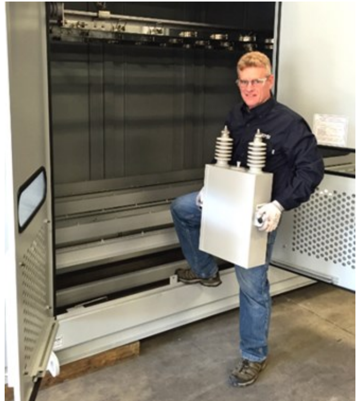
The ease and convenience of maintaining and repairing ground level equipment leads to short repair times and increased reliability
