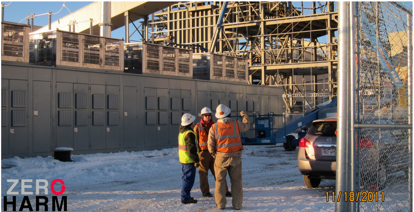
A large metal-enclosed harmonic filter system located at a large Copper concentrate plant in North America. NEPSI and NEPSI's harmonic filter systems embrace a 0-Harm policy. They are inherently safer, offer only controlled and safe access to live parts, reduce arc-flash hazards through numerous initiatives and design features, and prevent out-of-sequence operation.
